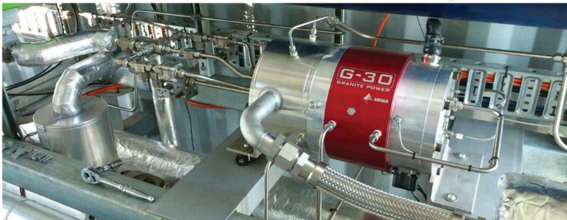
Figure 5 G-30 Turbine Installed at Wallsend
